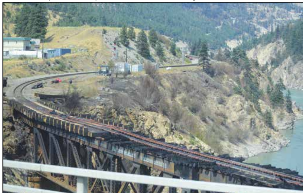
CN rail bridge over the Thompson River, July 9, 2021, showing burned rail ties. (Photo credit: Barbara Roden)
