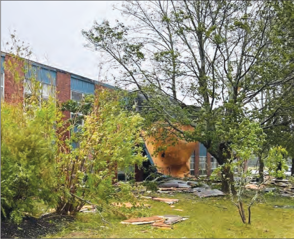
The front yard at Cardigan Consolidated School was covered in heavy debris after Fiona damaged the structure's roof. A satellite dish, at the front of the school hung precariously over the side of the building. Classes were cancelled Island-wide on Monday and Tuesday with another announcement expected about mid-week. The status of the Cardigan School wasn't known at press time.
