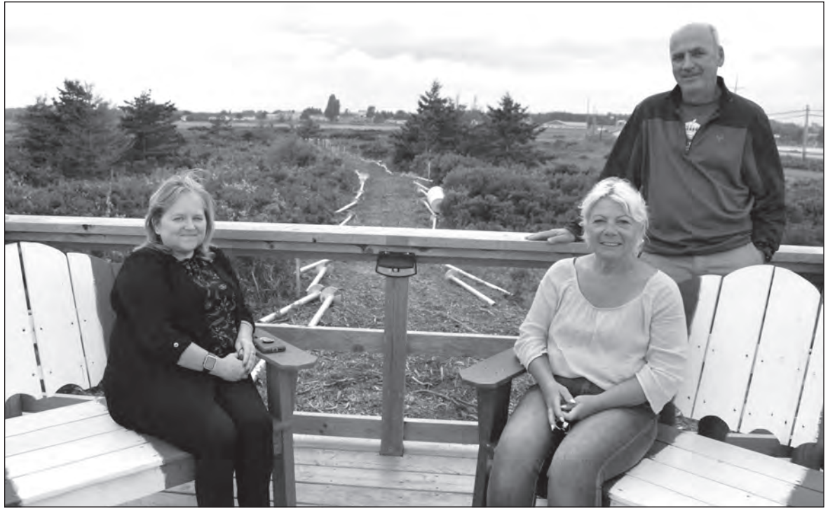
The installation of posts for the expansion to Souris Beach Boardwalk was in full swing last week when town officials CAO Shelley LaVie and Mayor Joanne Dunphy met with Friends of Souris Beach committee member Brian Deveau to talk about the progress. Charlotte MacAulay photo
