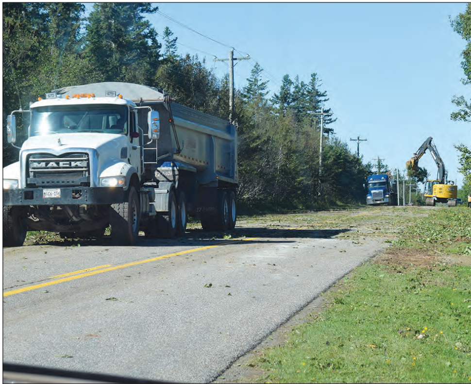
Crews were out on the North Side Road in Hermanville all day Sunday clearing downed trees. Dozens of dump truck loads of decimated trees were trucked away. Charlotte MacAulay photo
