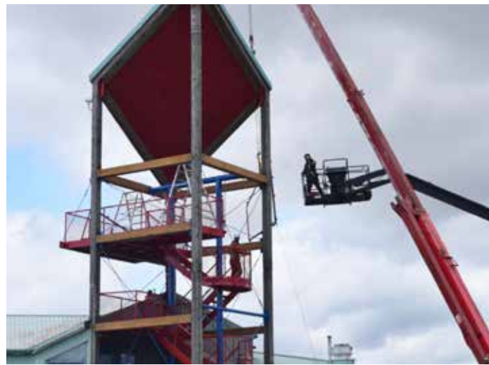
Contractors work on the Harbour Quay Story Tower on May 25, 2022. (ELENA RARDON / ALBERNI VALLEY NEWS)
