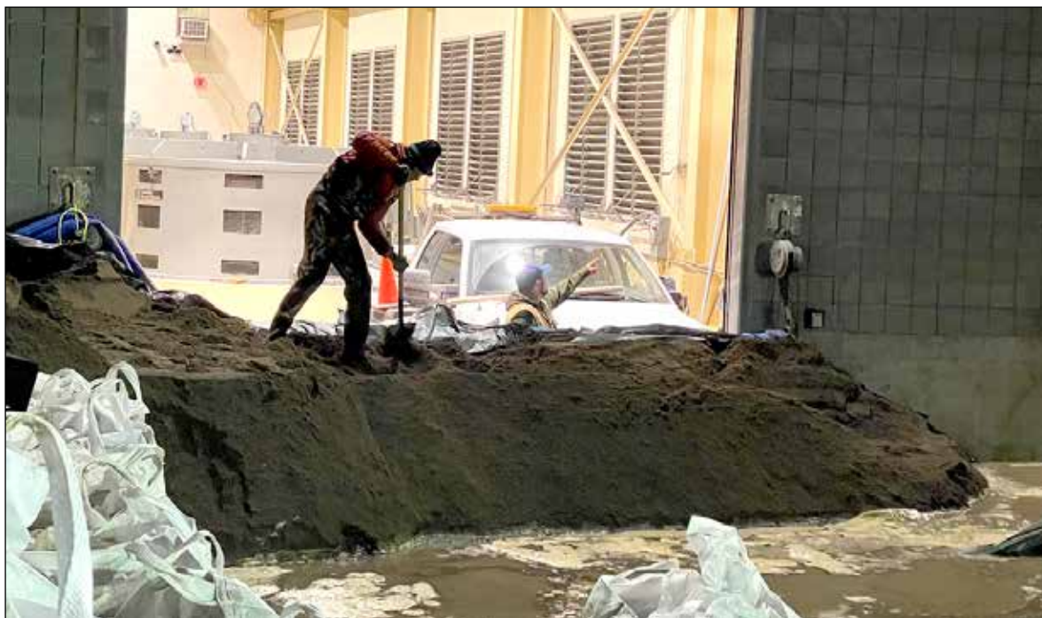
Chris Kitt at work surrounding the side door of the Barrowtown Pump Station in November 2021. (Submitted photo)
