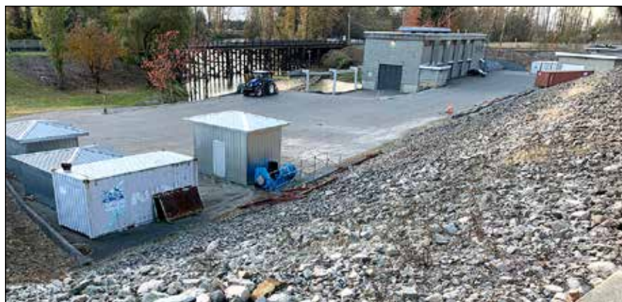
The Barrowtown Pump Station is back to normal operations, but was at the centre of the flooding disaster in Abbotsford in November 2021. (Jessica Peters/Abbotsford News)
