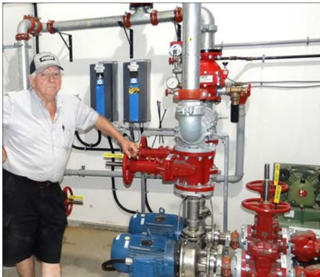
Gilmer Penner in the fire suppression equipment room at the new 305,000-square-foot Pennwood Dairy barn.
